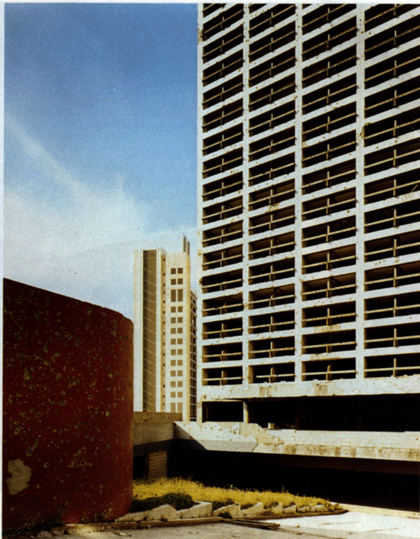
GHOSTS OF VACATIONS PAST The bullet-pocked walls of Beirut's old Holiday Inn testify to the damage inflicted on the city's buildings during Lebanon's civil war.
